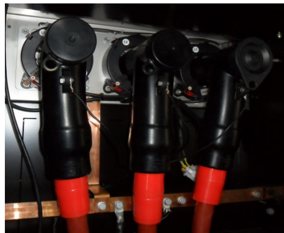
Real cable terminal configuration error (central cable) detected during energizing of the WTG. This kind of errors can be discovered by Partial Discharges monitoring prior to energizing.
