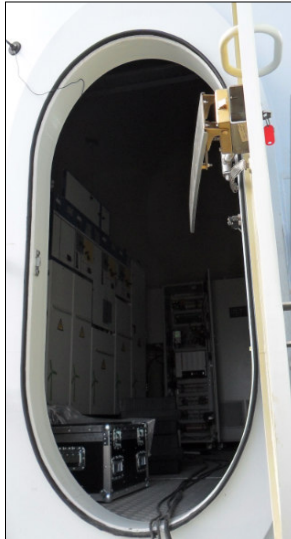
MV switchgear with integrated Protection & Control devices inside a WTG.
