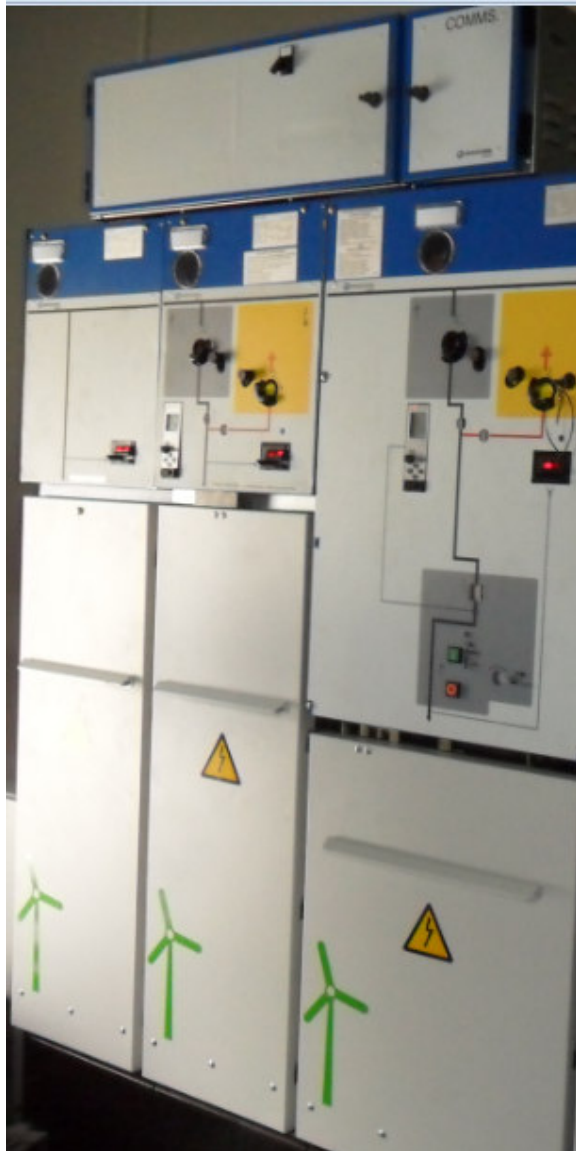
MV switchgear with integrated Protection & Control relays connected to the communications network to perform remote control and monitoring of the switchgear inside a WTG.
