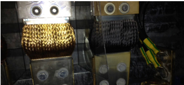
Accurate room temperature models can even help to detect overheated junctions
