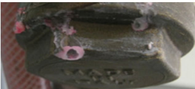
An almost invisible leak can cause a turbine stop over time. It can be detected by advance pressure models
