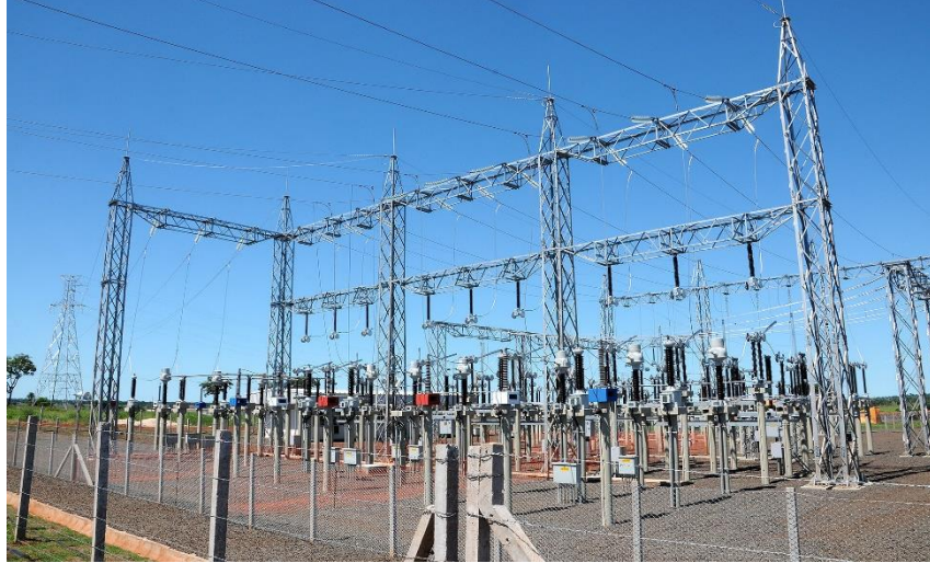
Alto Jahuel Substation
